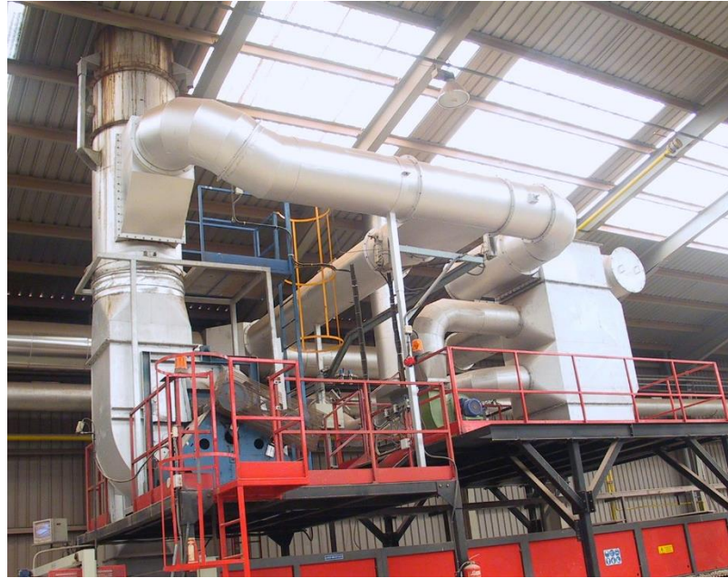
Figure 5. Flue gas/air heat exchanger installed in a kiln (Courtesy of Poppi Clementino, s.p.a.)
